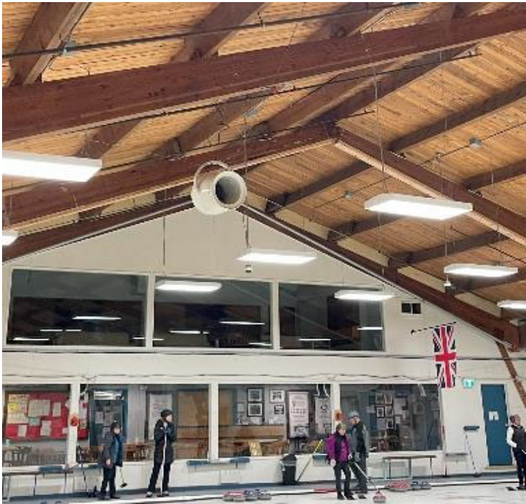
Fan located above curling rink ice surface
