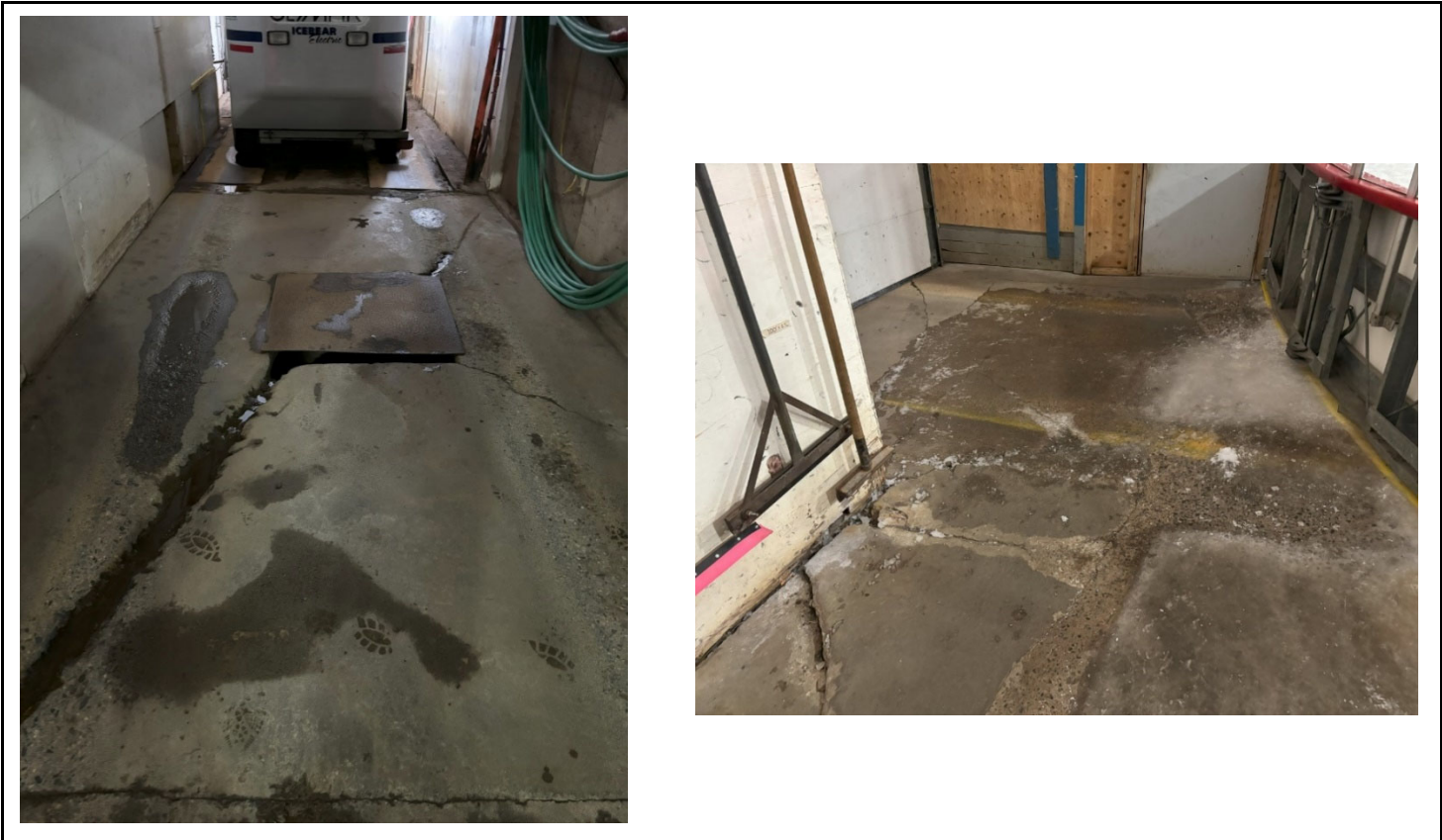
Damaged concrete slab at Zamboni ramp & Damaged concrete slab at Zamboni addition
