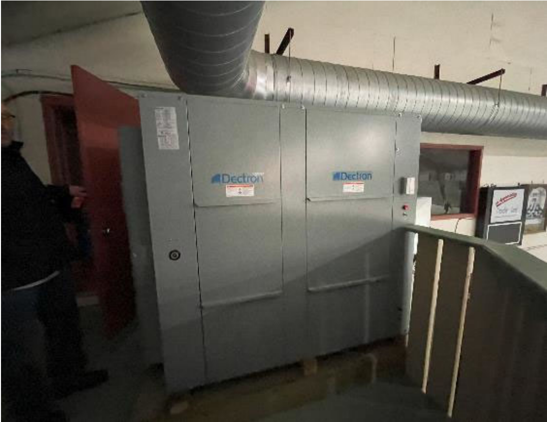
Dehumidifier unit serving hockey rink
