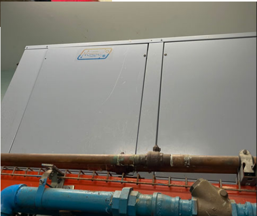
(Left) Two hot water tanks preheated from a heat pump. (Centre) Propane booster water heater. (Right): Heat Pump
