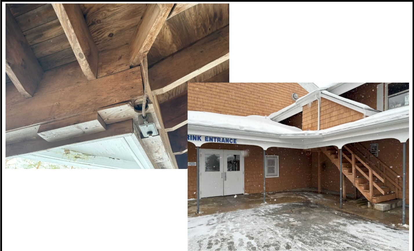
Canopy Structure at hockey arena entrance + Canopy Structure at hockey arena entrance with missing steel post
