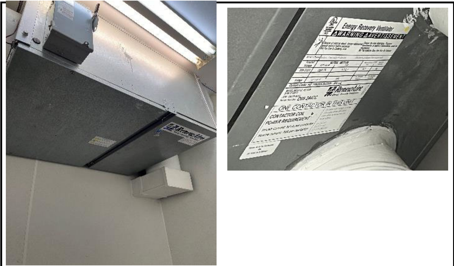
Energy recovery ventilator located outside locker room for hockey rink
