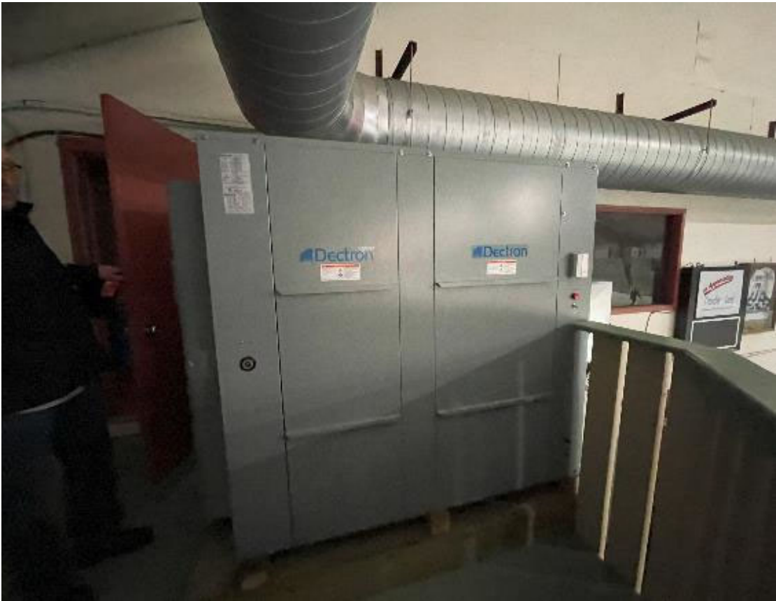
Dehumidifier unit serving hockey rink
