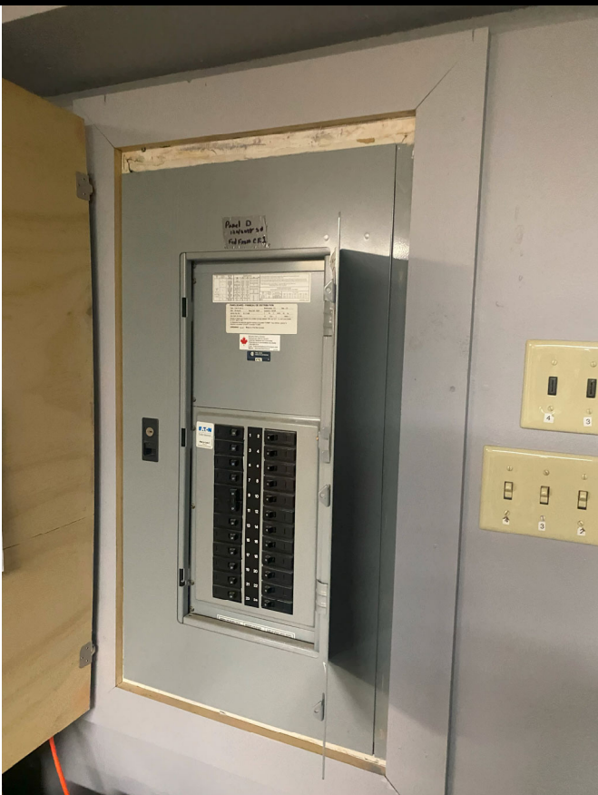
Branch Circuit Panelboard - Newer Style
