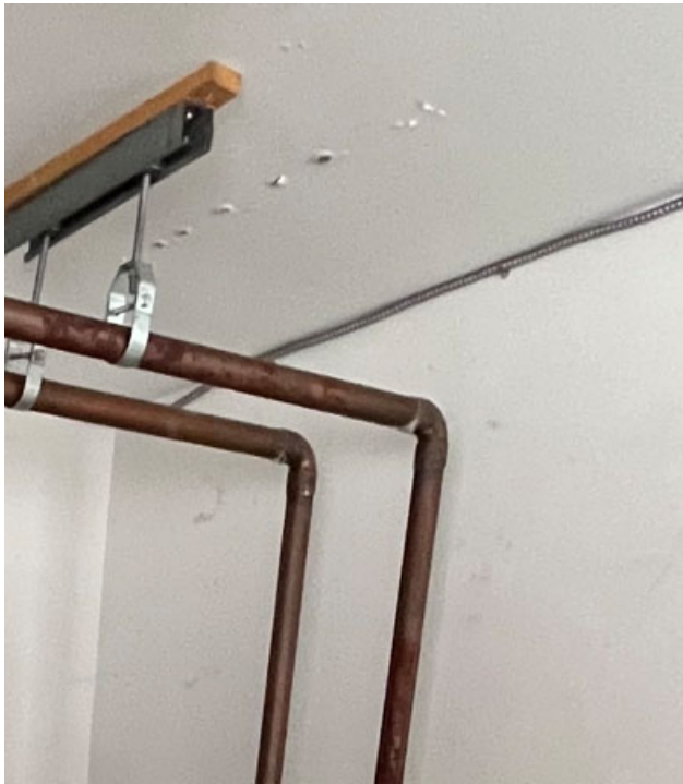
Copper Domestic Water Piping
