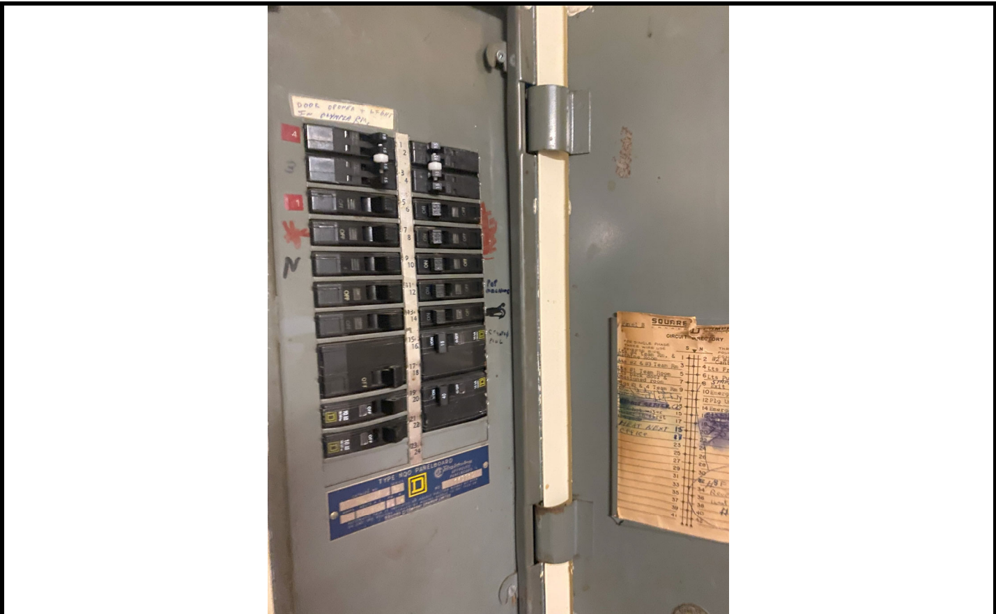
Branch Circuit Panelboard - Older Style
